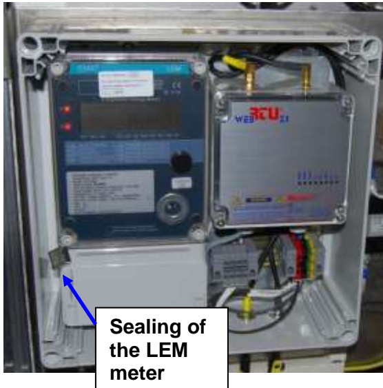
Detailed view of an EMU, showing sealing of the LEM meter.
