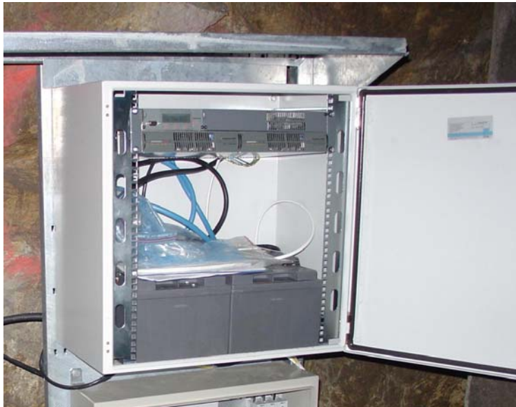
Figure 10: Rectifier and batteries in rack inside a tunnel
