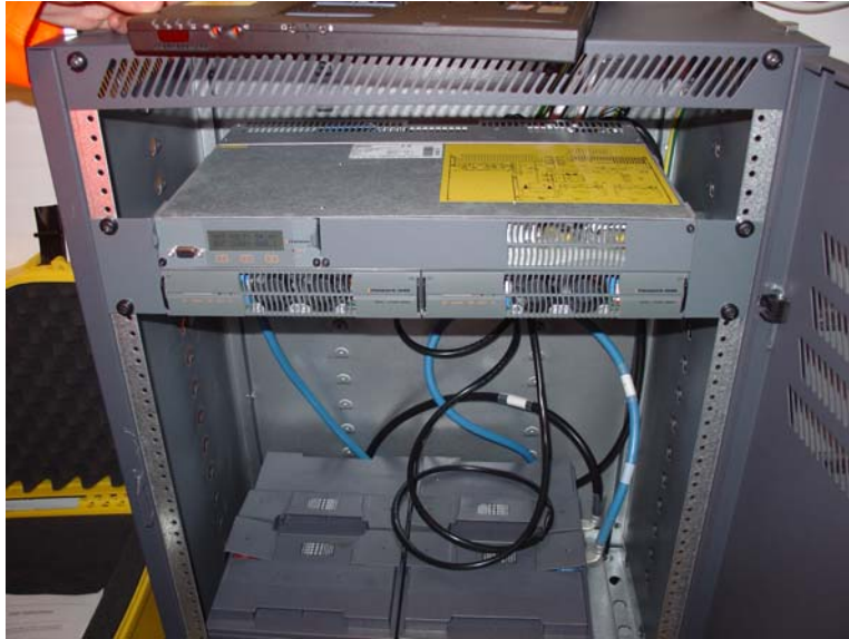
Figure 9: Rectifier and batteries in rack inside shelter.
